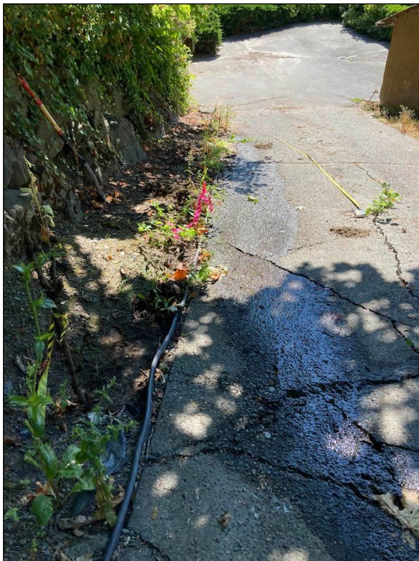
Photo 7. Seeps draining out of lower driveway adjacent to Wetland A (photo taken 7/23/21).
